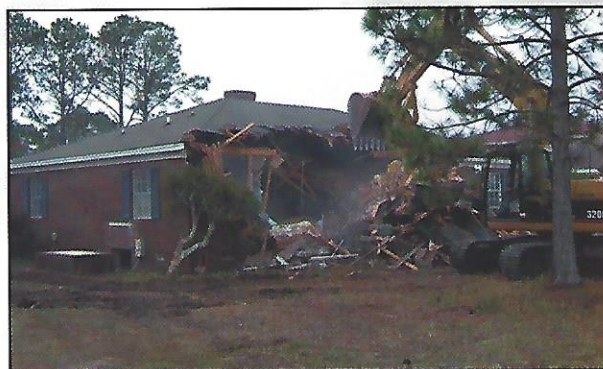
Home being demolished due to mold from water intrusion
